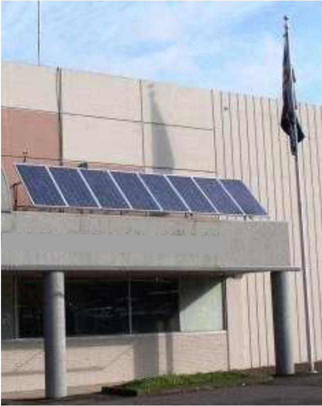
Fig. 1: Flagpole located to the east of a 1.3 kW photovoltaic system. The system is tilted at 45° and an azimuth of 200°, a little west of true south. The pyranometer is mounted on the top of the panels between the third and fourth panel from the east.
