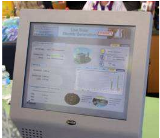
Kiosk showing kWhrs produced for viewing by Camping World customers
