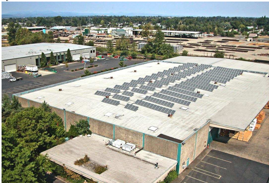
Fig. 1: 65 kW PV installation at West Wind Forest Products.
