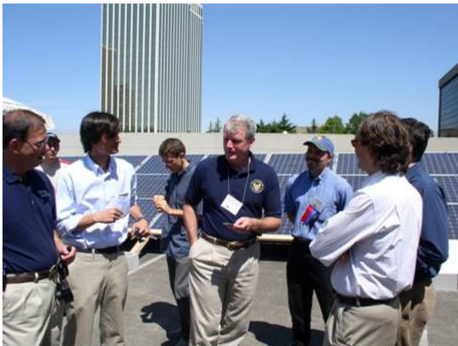
Congressman Brian Baird talking to a representatives from Isofoton with the Isofoton 6 kW photovoltaic array in the background.
