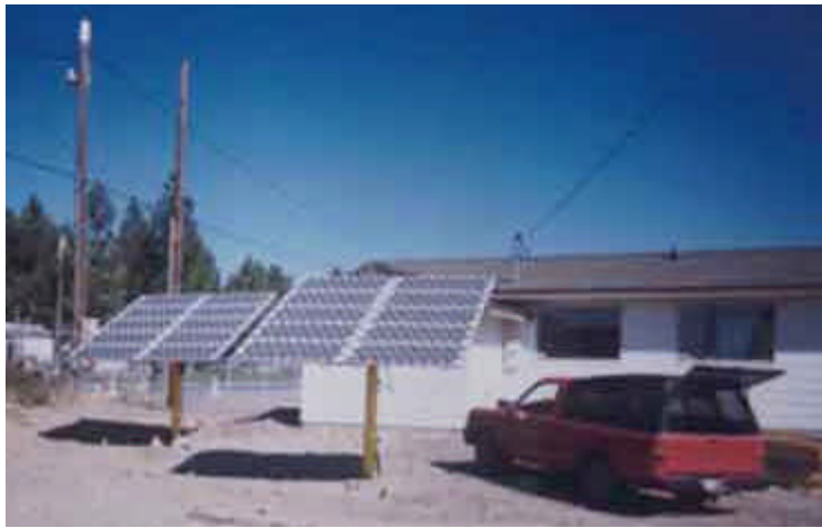
Two kW array outside Collins Pine Products
