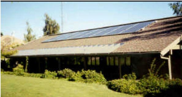
5kW solar cell array on the roof of Ashland's Civic Center. Note that the array fits in with the architecture of the building.
