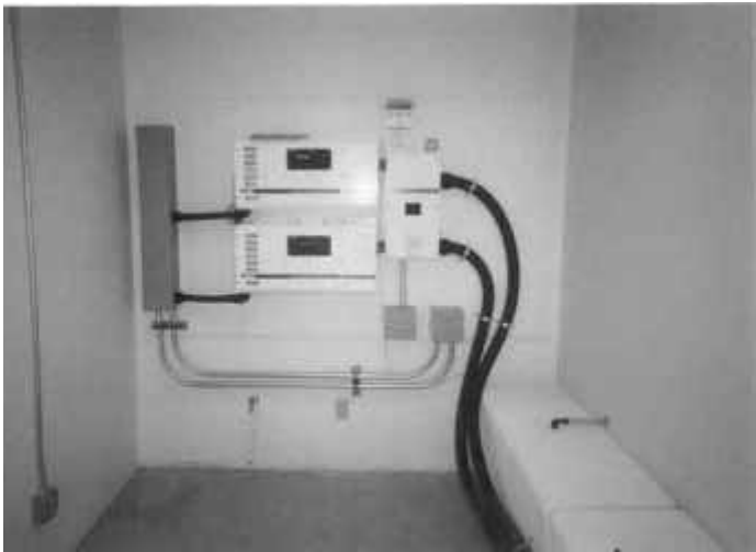
The stacked pair of Trace SW5548 sine wave inverters and two racks of Trojan L16 lead acid batteries
