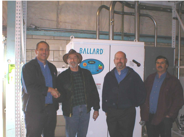
John Bocchi, David Parker, Steve Bocchi, and Toni Bocchi celebrating the installation of the solar electric system.
