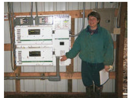
Ready to power up. Photo ESCO
