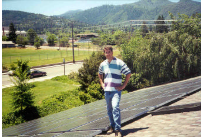
Tim McFail of Applied Power stands next to the 15 kW PV array installed on Ashland's police headquarters. A total of 25 kW is being installed in the first phase of the Ashland Project.
