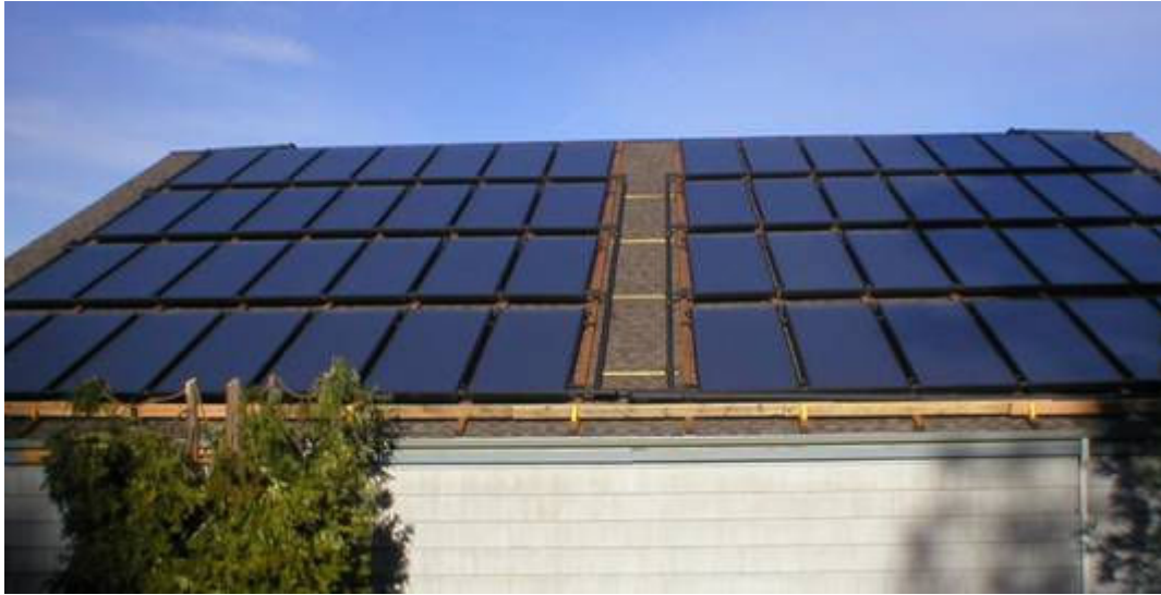
Tamarack Wellness Center Commercial Hot Water and Pool Heating System: A total of 56 solar water heating panels supplies feeds a 600 gallon tank.
