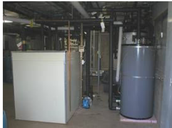
Tamarack Wellness Center pool 600 gallon tank with Voyager
